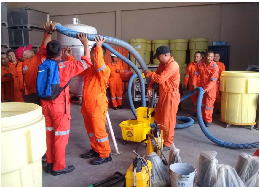
Pemasangan peralatan oil spill vacuum system / Installation of oil spill vacuum system.
